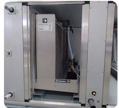
Example of an FA6 installation in a section of an airhandling unit.
